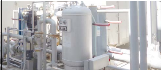
An environment-friendly co-generation system using natural gas at our Gunma Factory.
